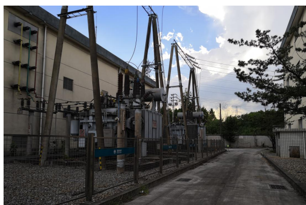
110kV 龚塘变电站现有主变
